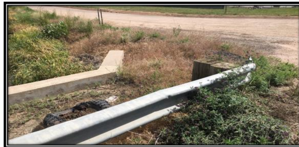
FIGURE 23: MINOR BEND TO GUARDRAIL IN THE WESTBOUND SIDE
