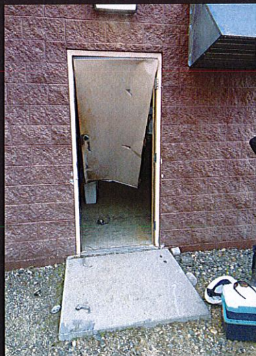
Break-in at South Tank Site pump station
