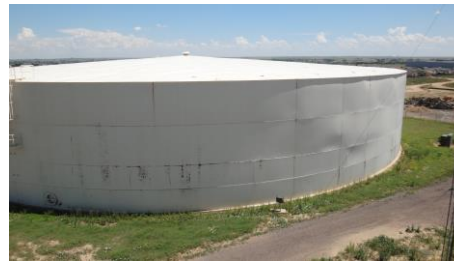
8,300,000 gallon ground reservoir
