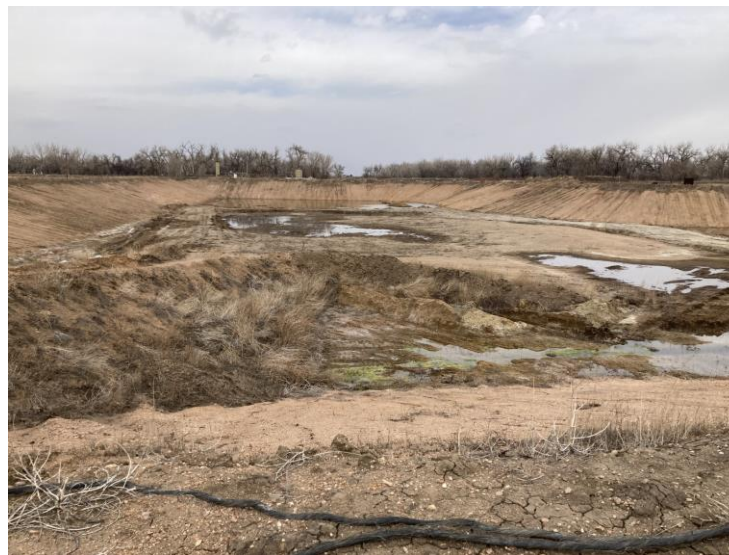
New Storage Reservoir
