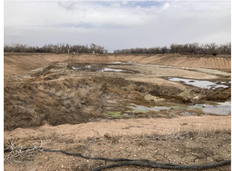
New Storage Reservoir
