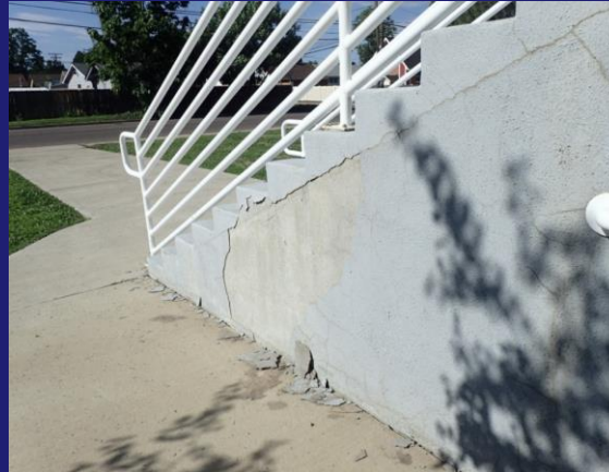
Extent of structural deterioration on original building (bottom two photos)
