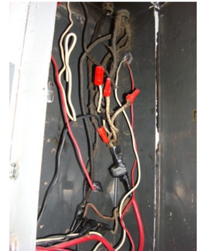
Basement branch circuit wiring
