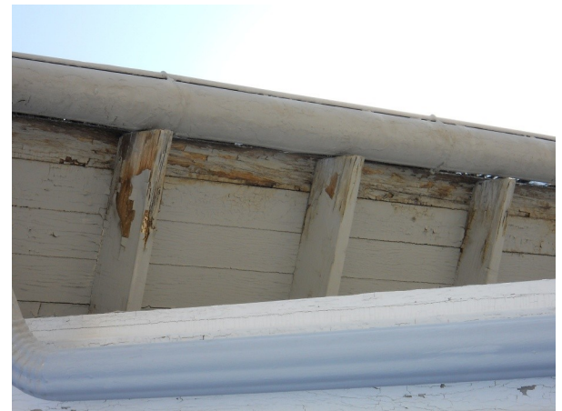
Deteriorated sheathing and rafters at west porch
