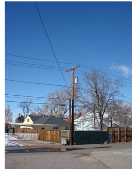
Telephone Overhead Service
