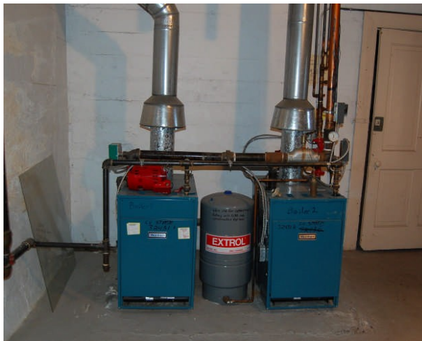
Basement Level Boiler System
