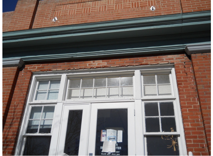
Damaged brick at south entry
