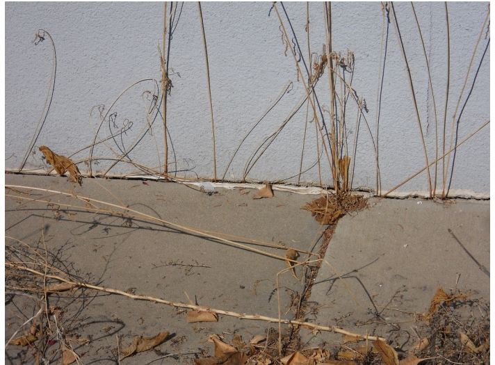
Deteriorated sealant joint at grade
