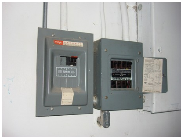
100A Panelboard (Basement)
