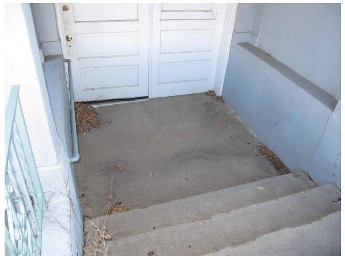
West exterior stairwell lacks an area drain.
