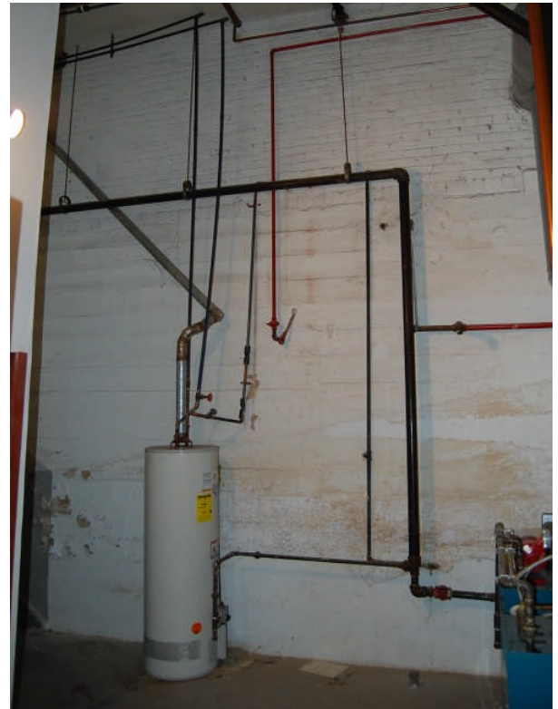
Domestic water heater
