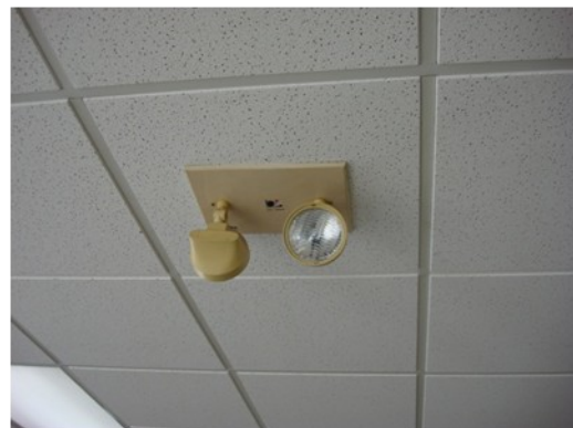
Typical EM Egress fixture
