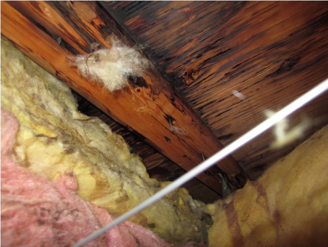
Roof deck deterioration where leaks in the roofing have occurred
