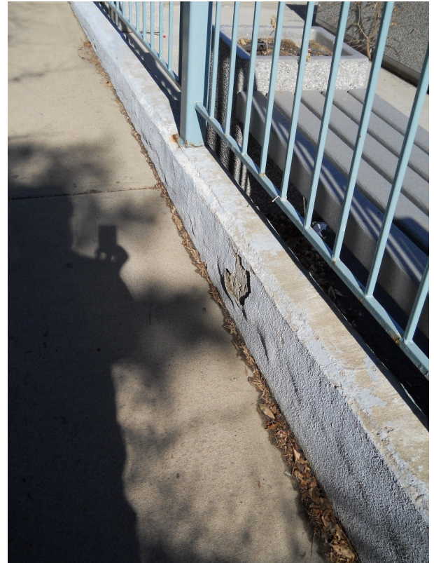
Deteriorated coating at east entry ramp
