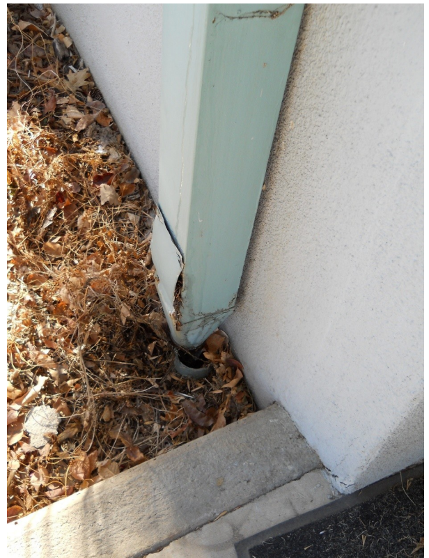
Downspout not connected to underground drain
