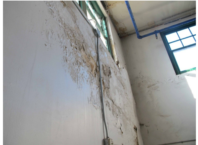
Deterioration of parge coat at interior face of foundation walls
