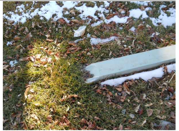
Crushed downspout extension
