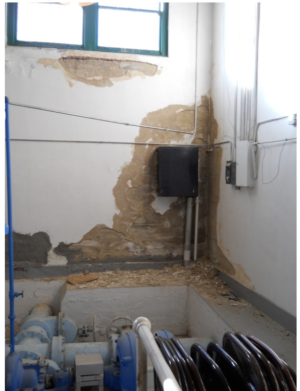
Deteriorated wall finish at basement
