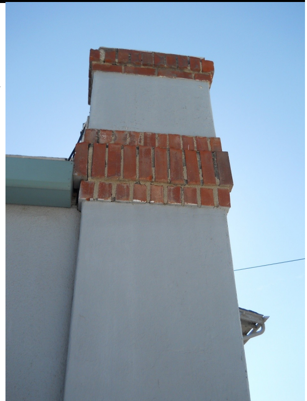
Deteriorated mortar joints and stucco at north wing
