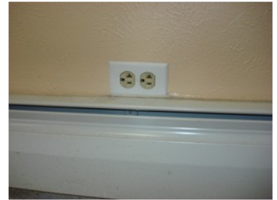
Receptacle Above Baseboard Heater
