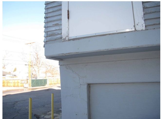
Cracking at concrete framing under the west balcony
