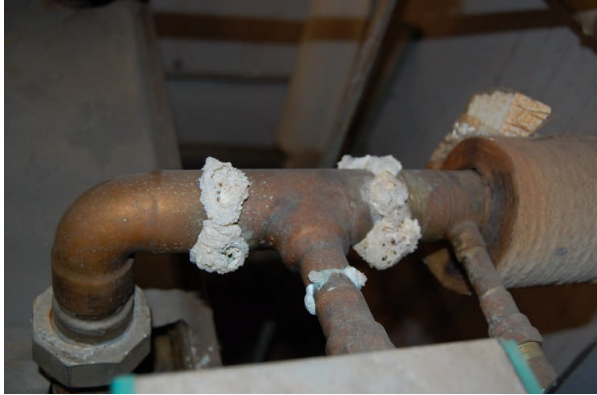
Main level corrosion
