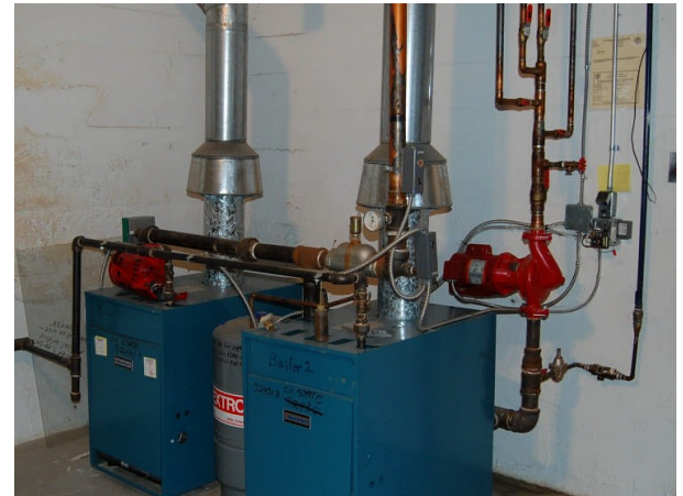
Basement pump and air scoop
