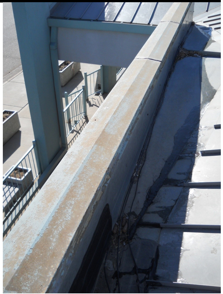
Corrosion at sheet metal coping
