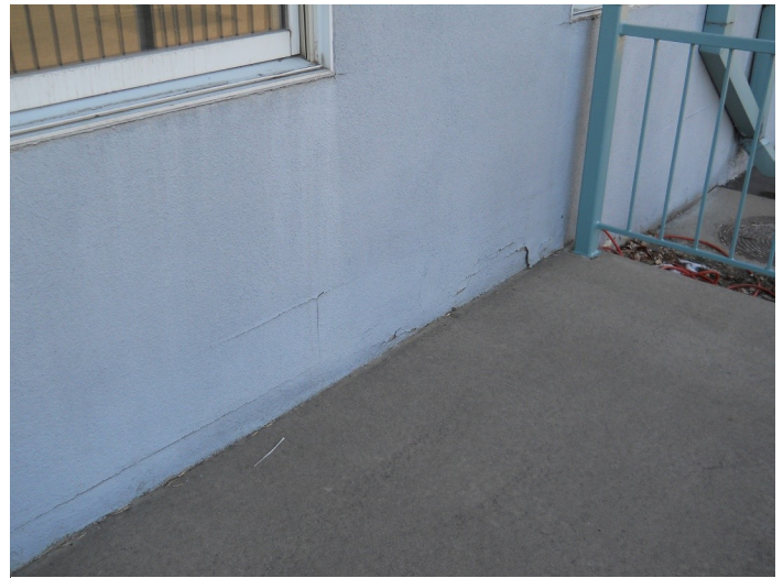
Cracks in EIFS at 1986 addition
