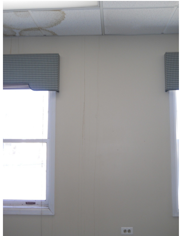
Water stains at dining room walls
