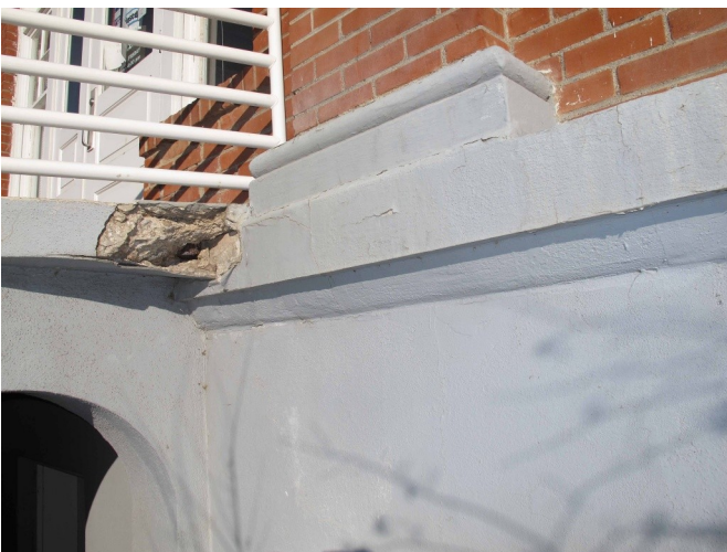
Concrete deterioration and cracking at the south entry stair landing
