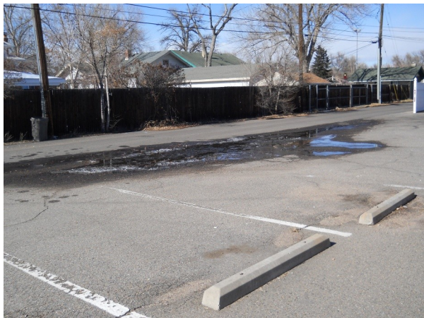
Ponding in parking lot
