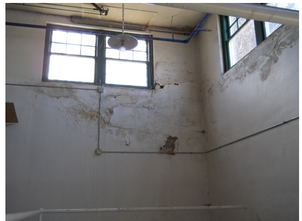
Deteriorated wall finish at basement
