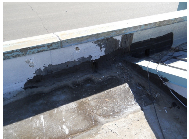
Repeated patching at scupper on 1986 addition
