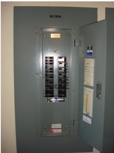
100A Panelboard 'LP1'
