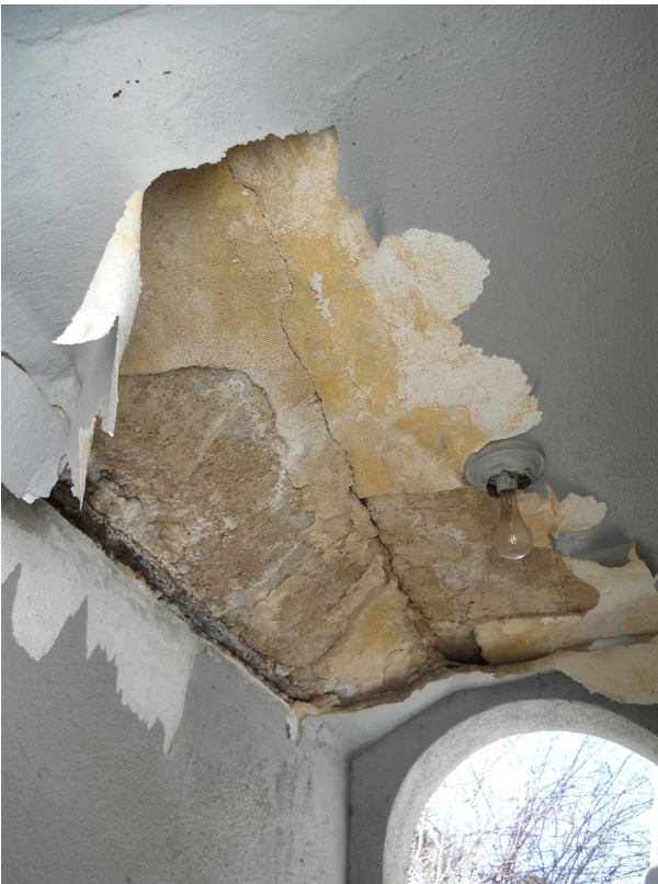
Concrete slab deterioration at south entry landing
