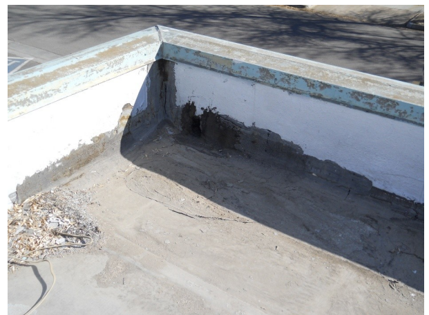
Repeated patching at scupper on 1986 addition
