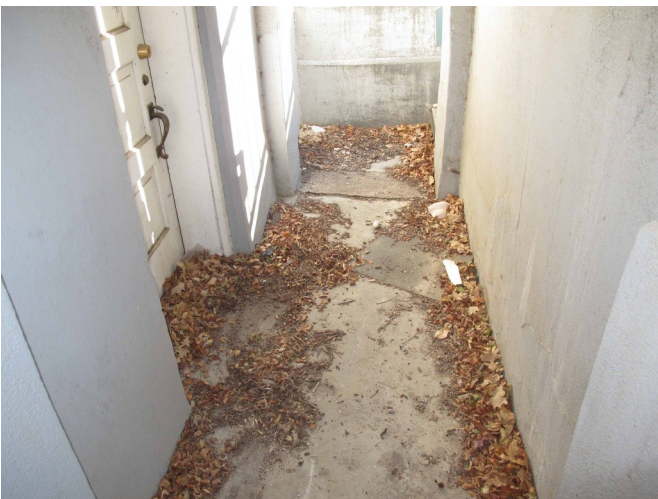
South exterior stairwell lacks an area drain.
