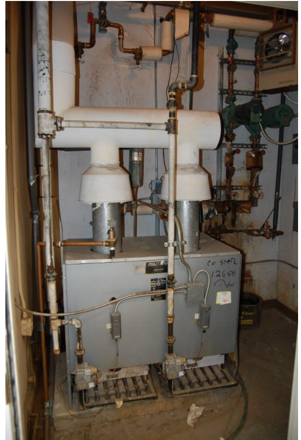
Main Level Boiler System
