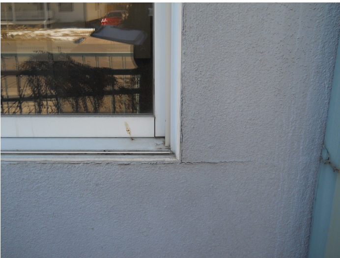
Cracks in EIFS at 1986 addition
