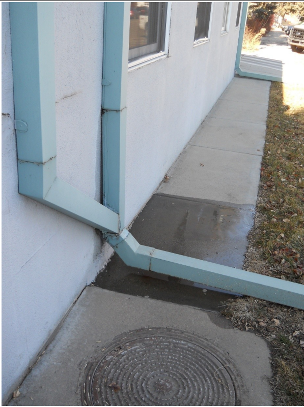
Leaking downspout and ponding water at north side of east entry
