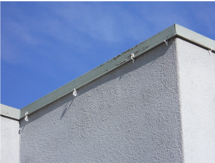
Failing paint at metal coping
