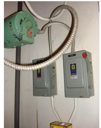
Mechanical Equipment Disconnects – Kitchen Mechanical room
