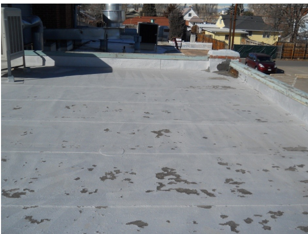
Failing coating on roof of 1986 addition
