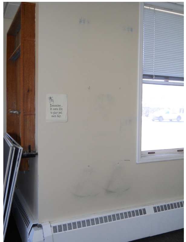
Damaged walls at billiards room
