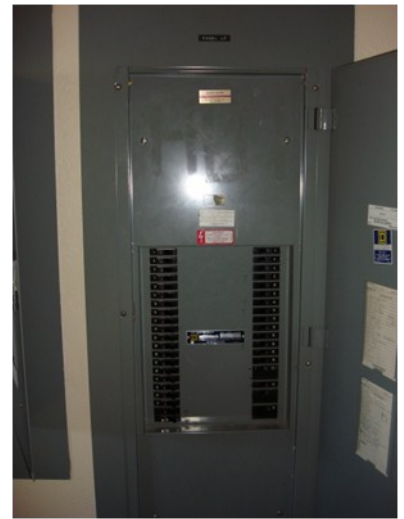
400A Panelboard 'LP'
