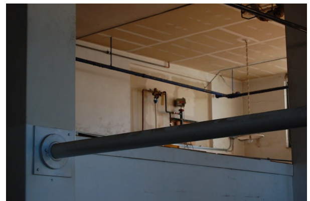
Domestic water backflow device
