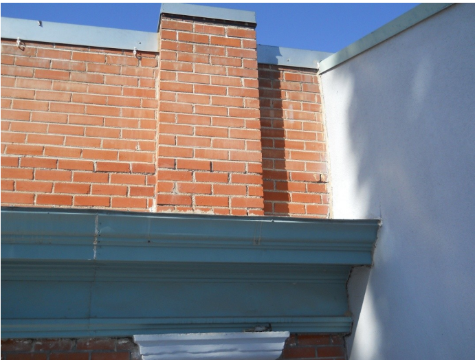
Deteriorated mortar at original building
