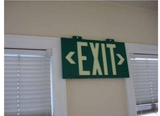
Non-Illuminated Exit Sign
