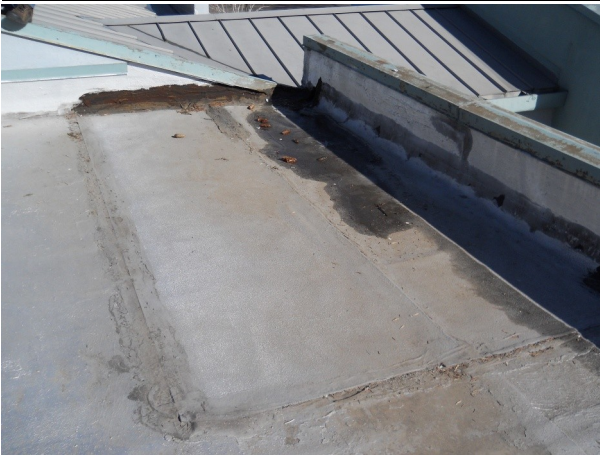
Ponding at scupper on 1986 addition
