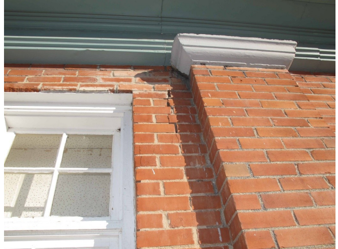
Deterioration of mortar joints
