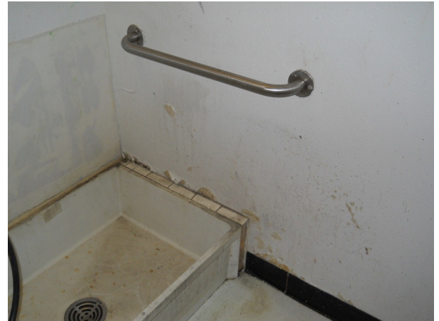
Drywall damage at upper level janitor closet
