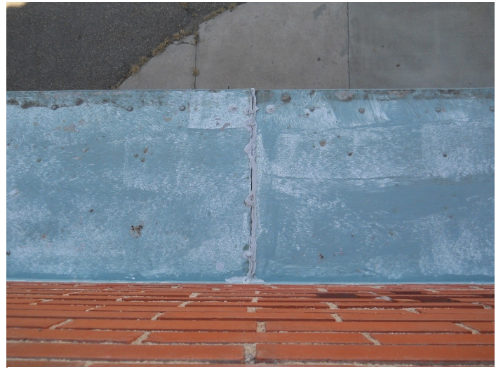
Joint on top of sheet metal cornice
