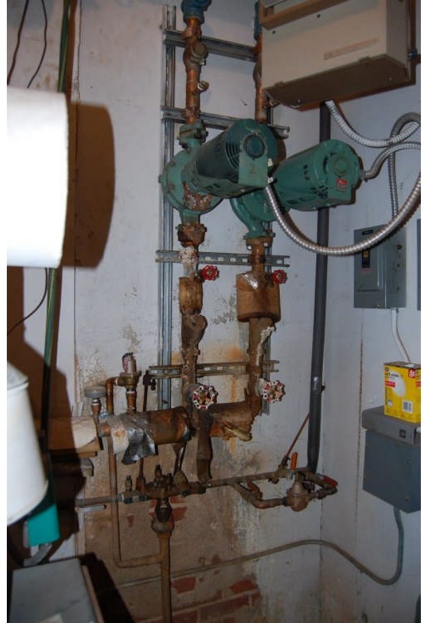
Main level pumps
