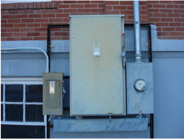
Wireway, Meter and Disconnects
