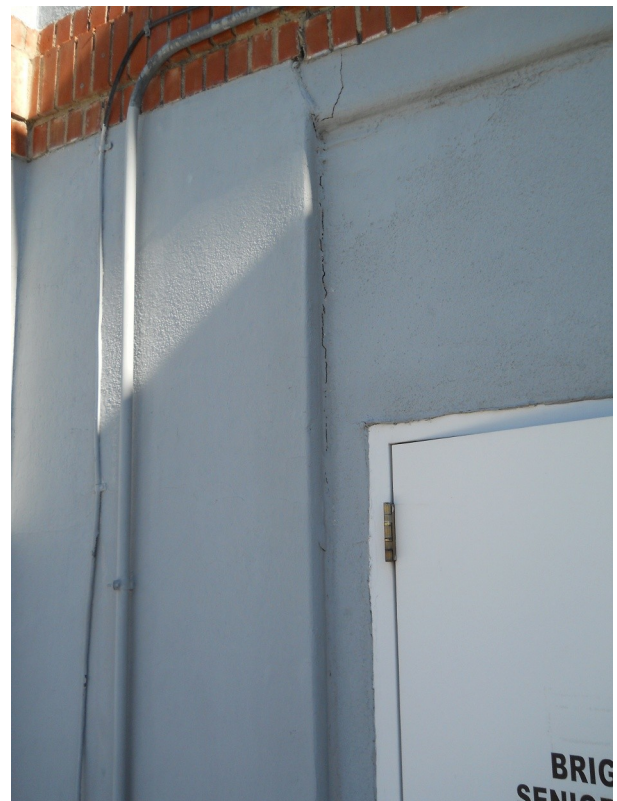
Deteriorated stucco at north wing
