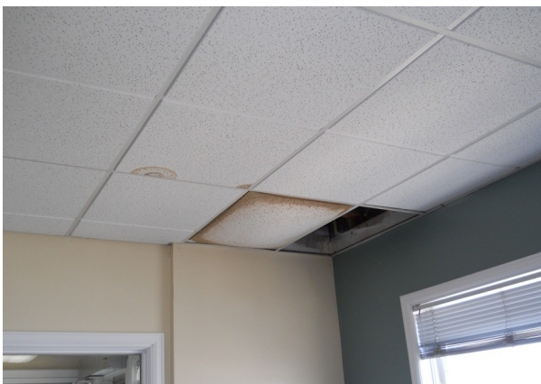
Water damaged ceiling tile
