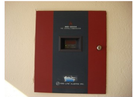
Fire Alarm Control Panel
