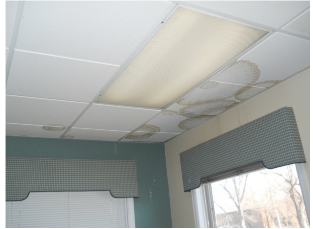
Water damaged ceiling tiles
