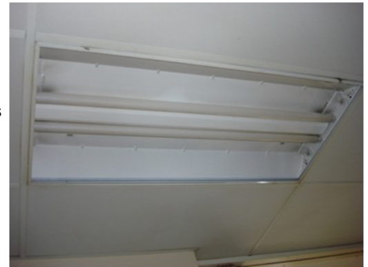
Damaged light fixture in kitchen
