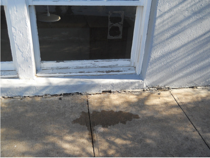
Deteriorated parking at grade
