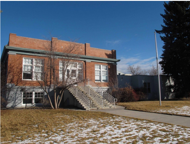
Site lacks positive drainage away from the building
