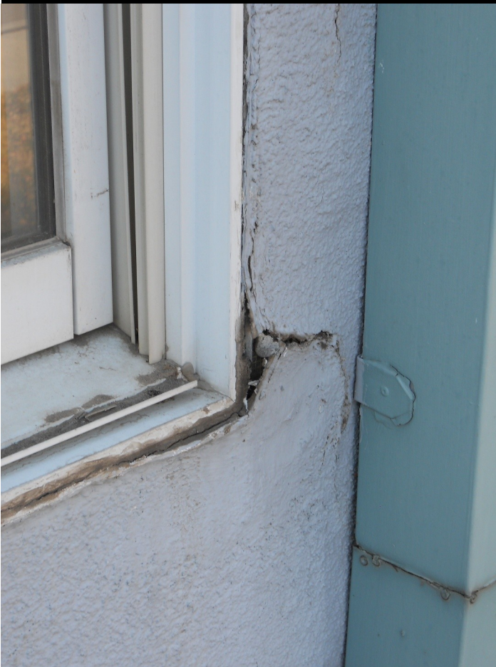
Cracks in EIFS at 1986 addition
