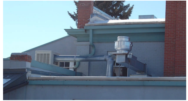
Kitchen hood exhaust and make-up unit
