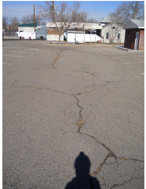
Cracked pavement at parking lot
