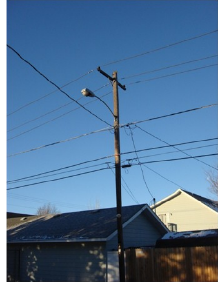
Overhead Electrical Service
