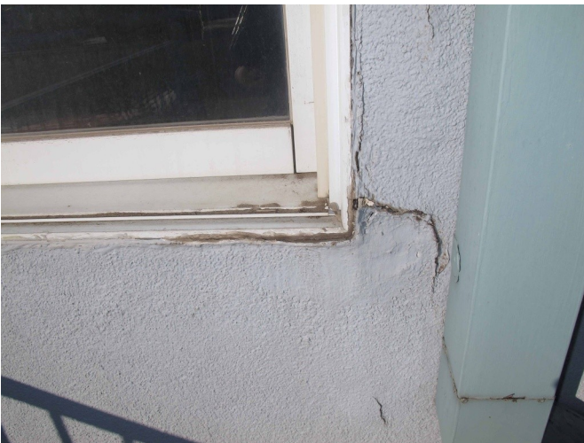
Cracking in the EIFS at the 1986 addition
