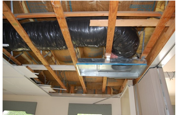
Interior ductwork in 2024
