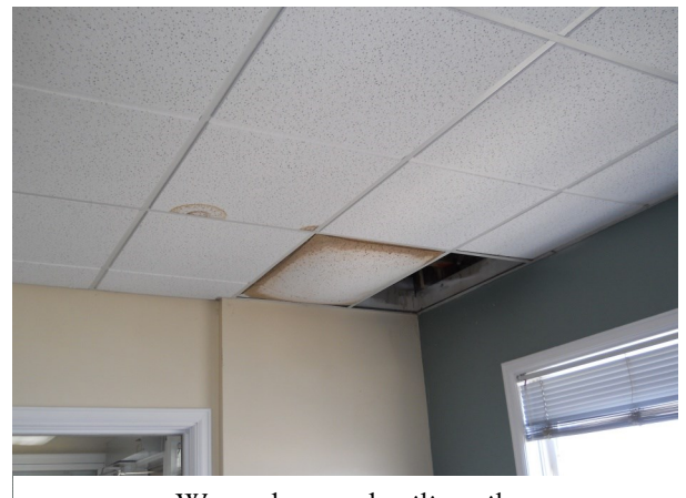
Water-damaged ceiling tile
