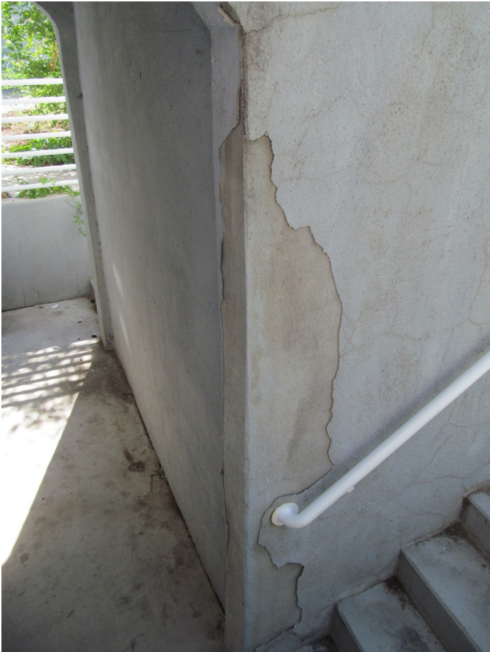
Delaminating parge coat at south stairs
