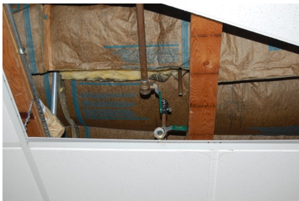
Main level piping in 2024
