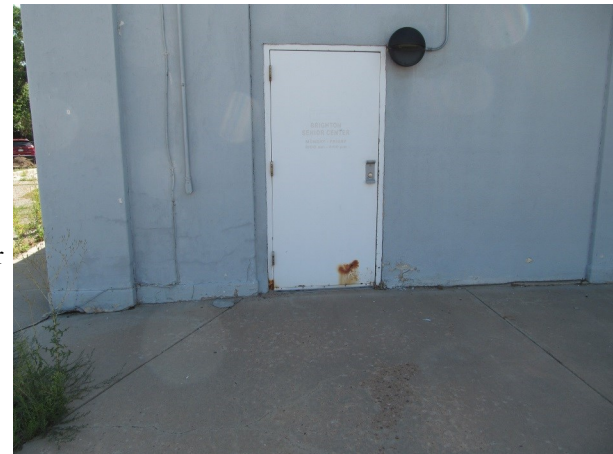
Deteriorated stucco at north wing
