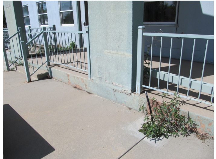
Deteriorated EIFS at east porch
