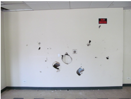
Vandalism damage at dining room wall
