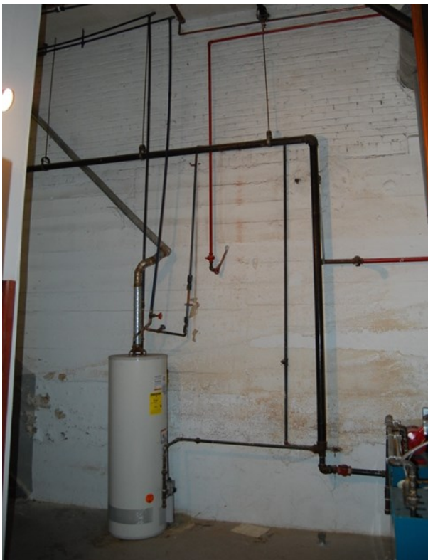
Domestic water heater in 2013
