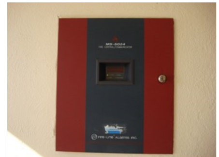
Fire alarm control panel
