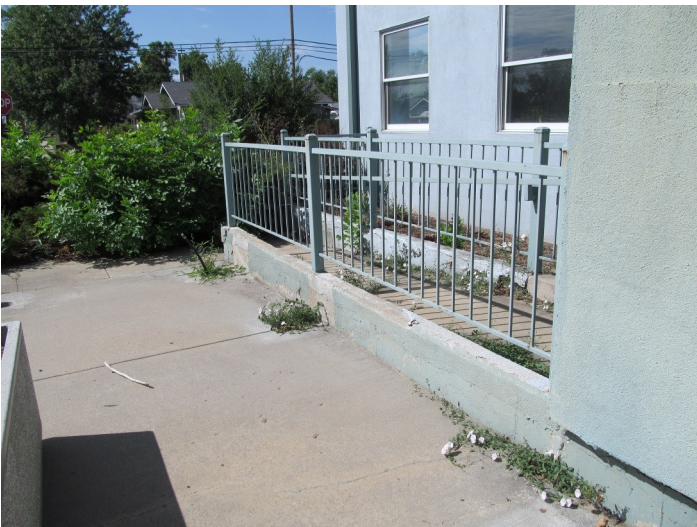
Deteriorated coating at east entry ramp
