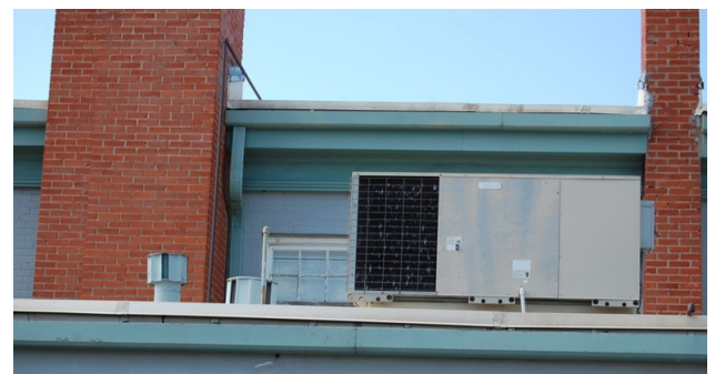
Kitchen area RTU in 2024
