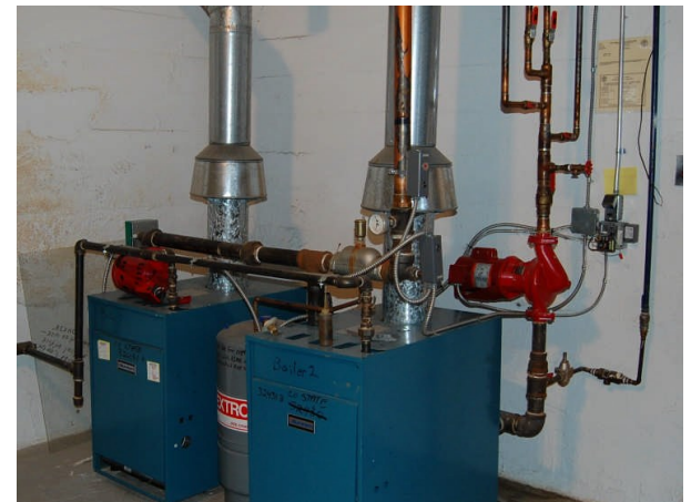
Basement boilers, pump, and air scoop in 2013
