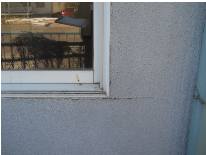
Cracks in EIFS at 1986 addition
