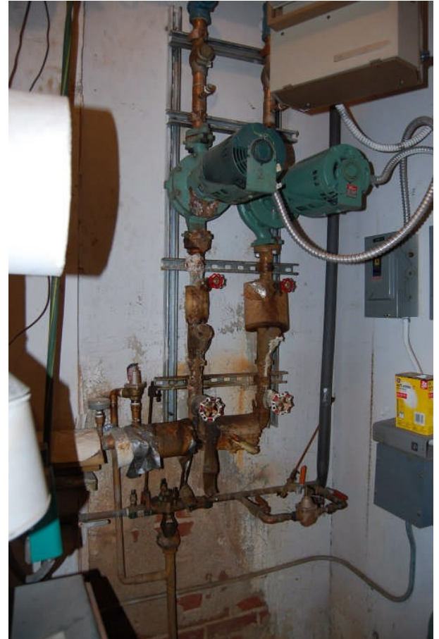
Main level pumps in 2013
