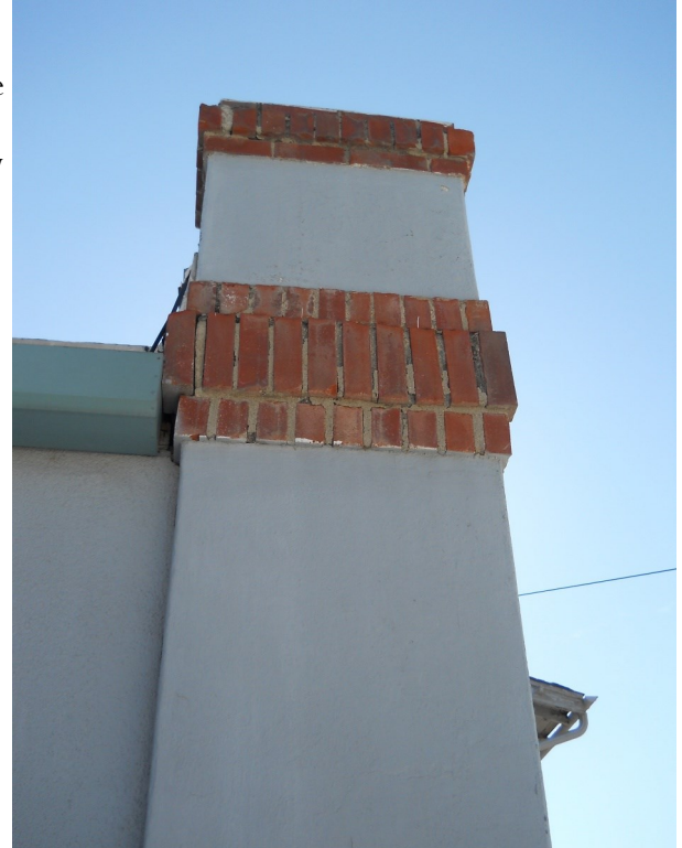
Deteriorated mortar joints and stucco at north wing
