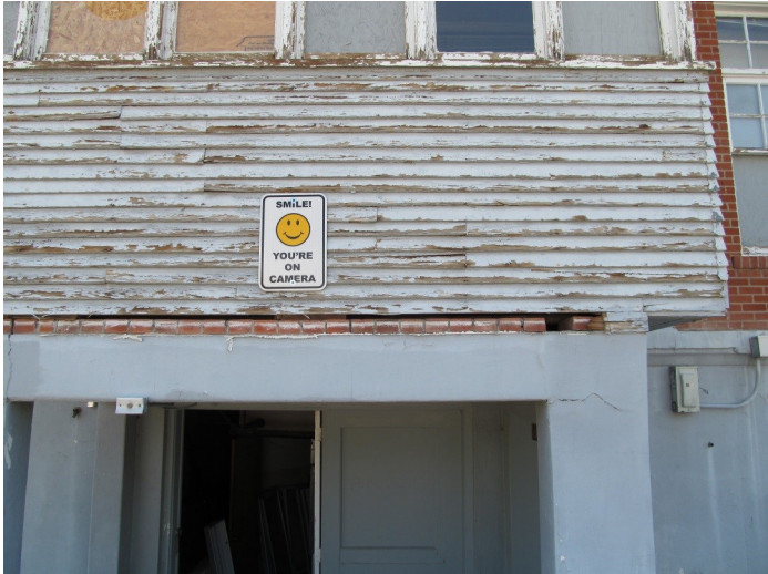
Deteriorated paint on siding at west porch
