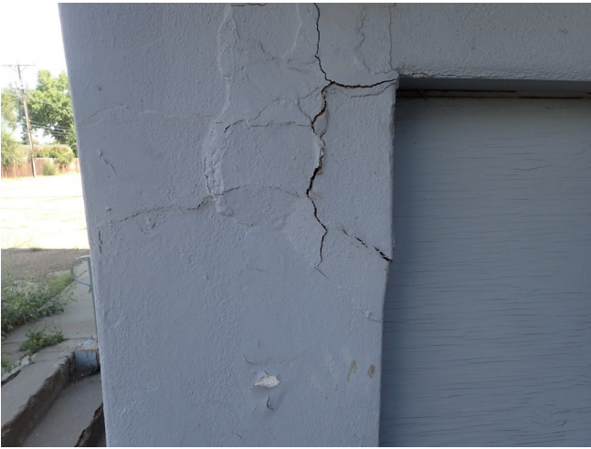
Failing bearing at enclosed balcony
