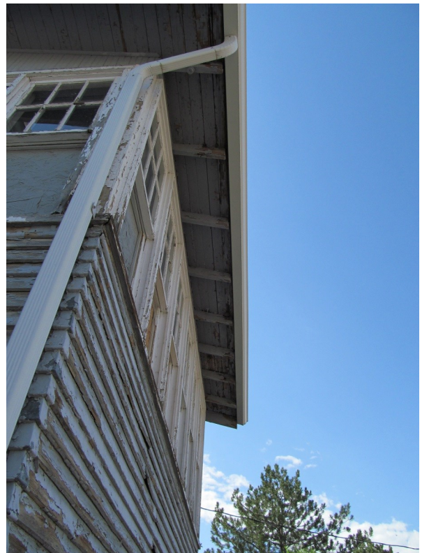
Deteriorated sheathing and rafters at west porch
