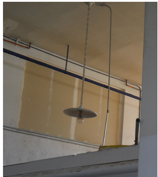
Basement light fixture
