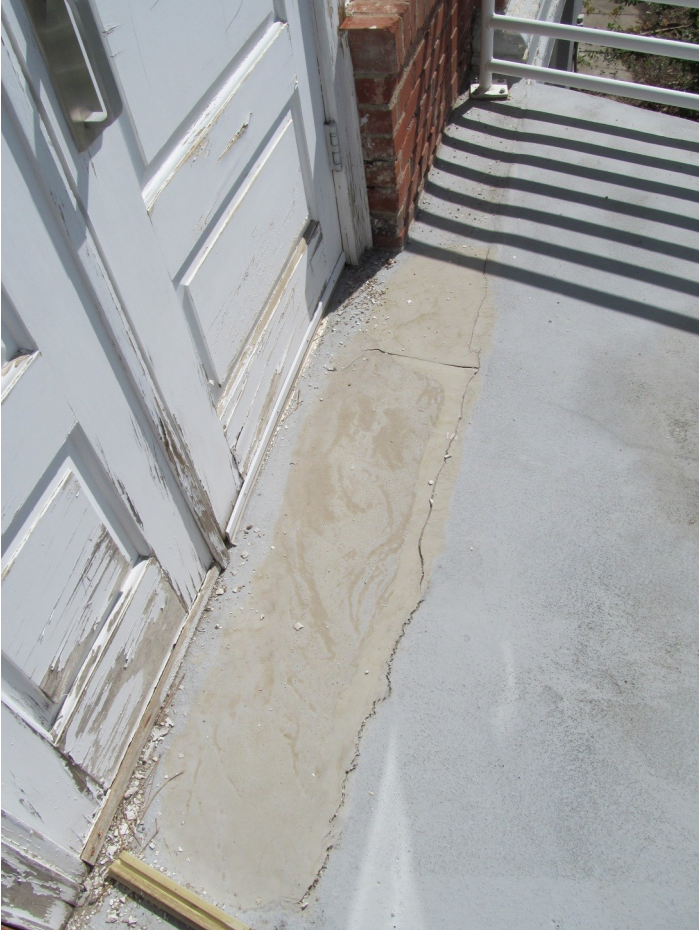
Cracks at south landing
