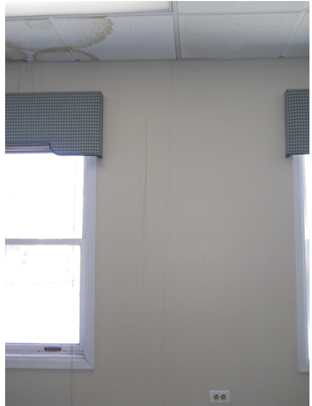
Water damage at dining room wall
