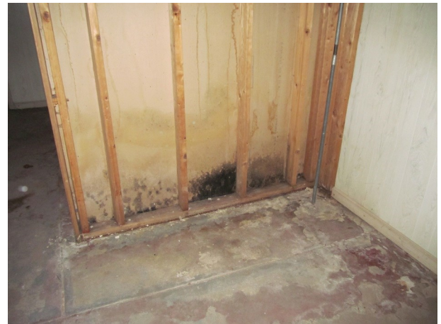
Suspected mold in basement
