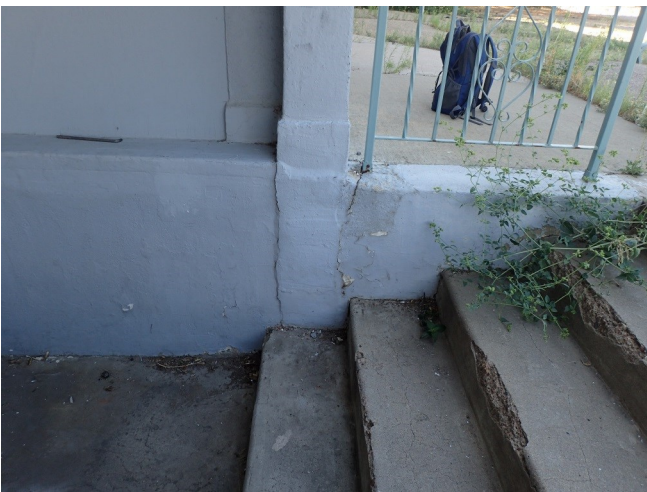
Base of south column at enclosed balcony
