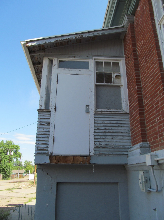
Damaged trim at west porch
