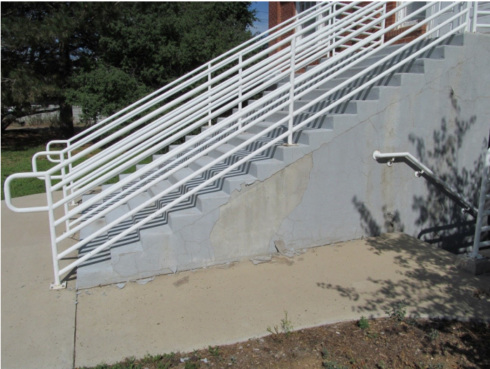
Delaminating parge coat at south stairs
