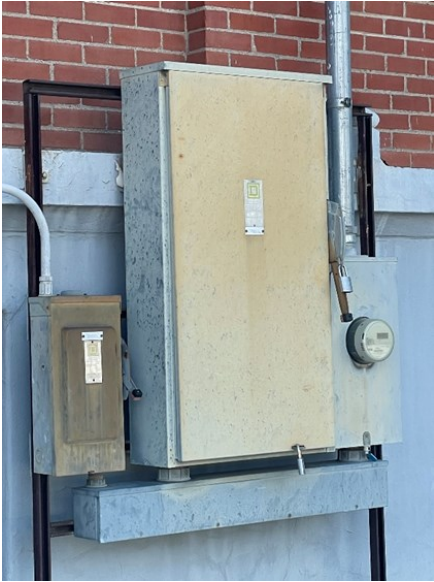
Wireway, meter and disconnects
