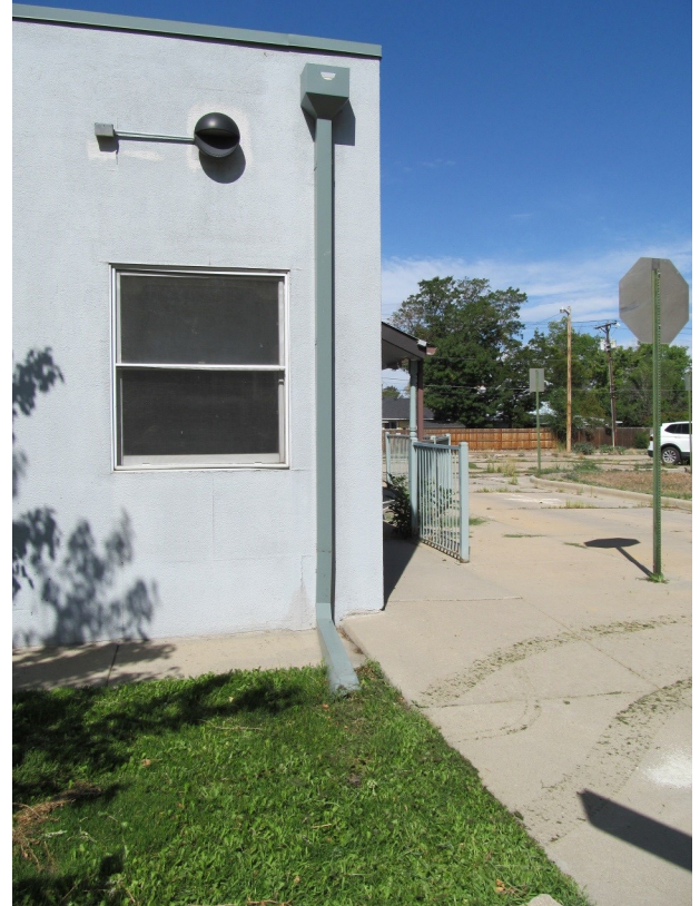
Crushed downspout extension
