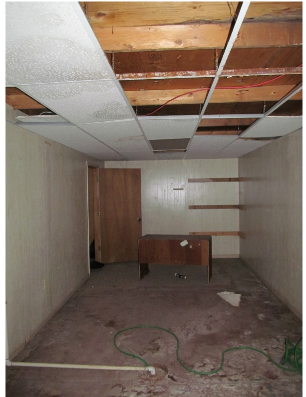
Water damaged ceiling at basement
