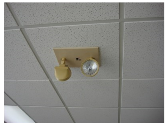
Typical EM egress fixture
