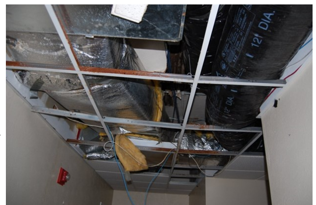
Interior ductwork in 2024
