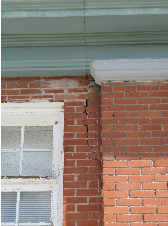
Cracks in brick wall
