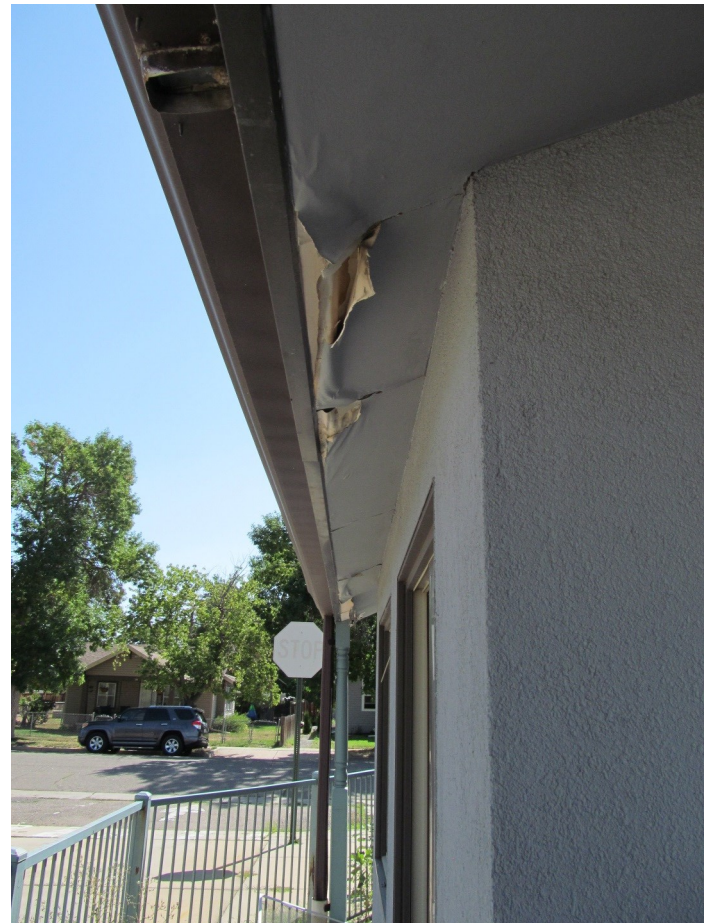
Water damage at soffit on north entry
