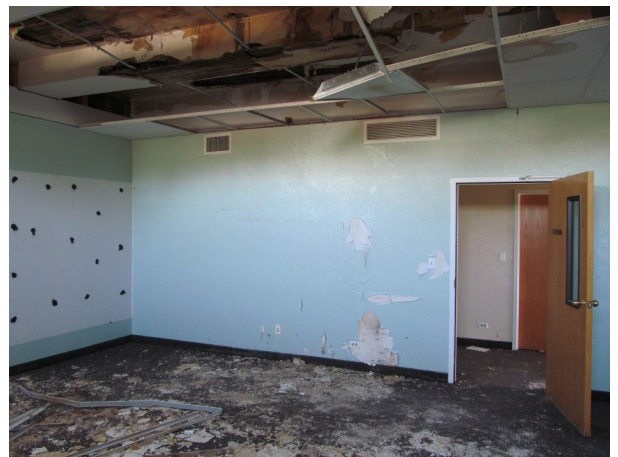
Drywall damage at upper level
