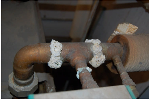
Main level corrosion in 2013
