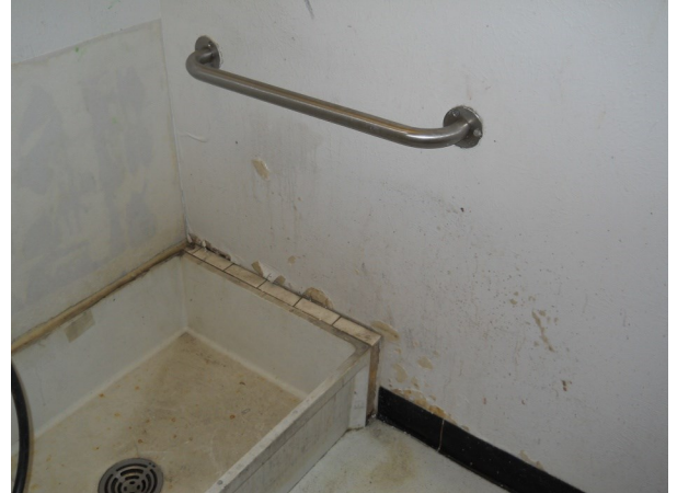
Drywall damage at upper level janitor closet
