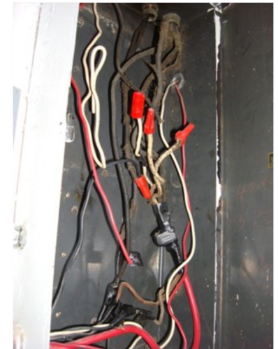
Basement branch circuit wiring
