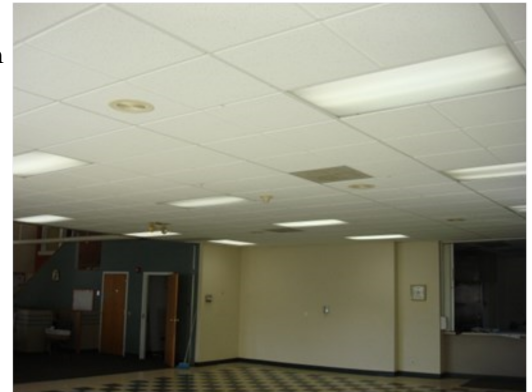
Typical fluorescent fixtures
