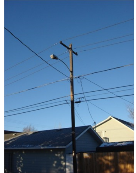
Overhead electrical service
