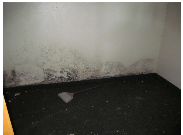
Suspected mold at upper level
