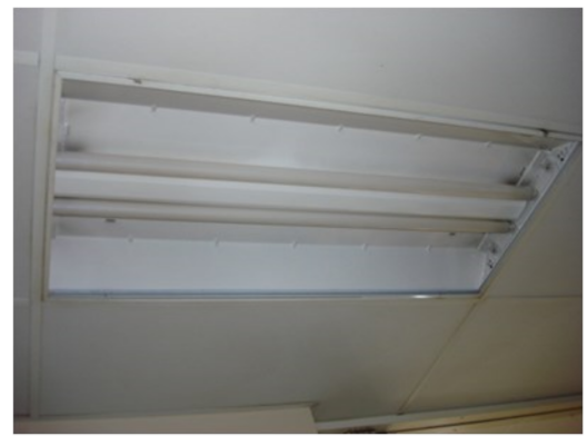
Damaged light fixture in kitchen
