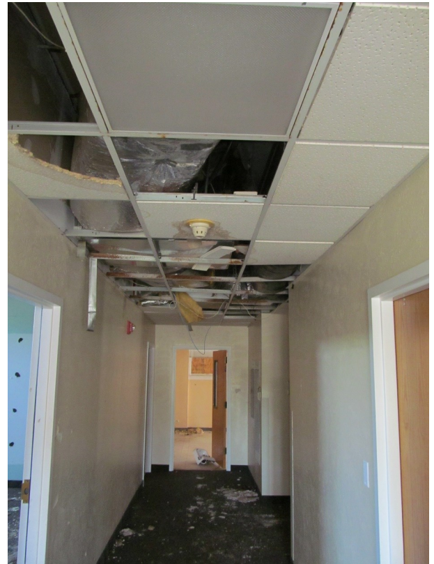
Ceiling damage at upper level
