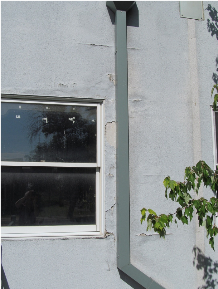
Cracks in EIFS at 1986 addition
