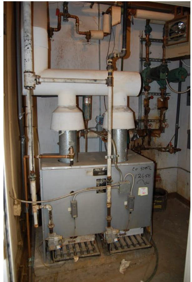
Main level boiler system in 2013
