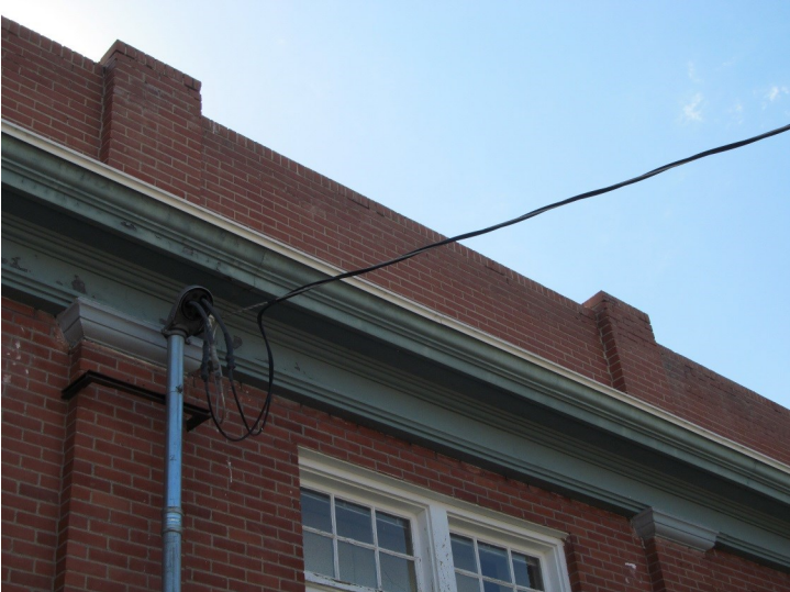
Peeling paint at sheet metal cornice
