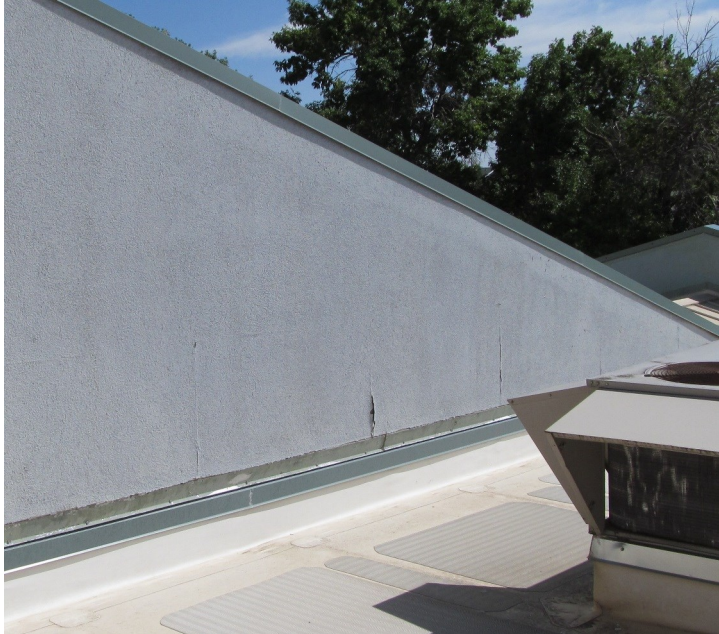
Cracked EIFS on 1986 addition
