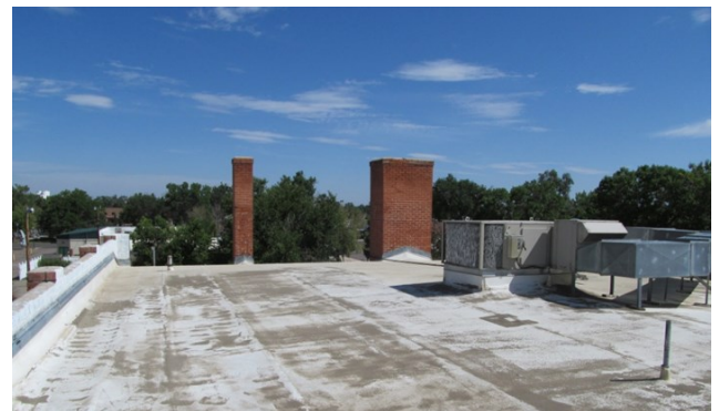
Upper roof RTU in 2024
