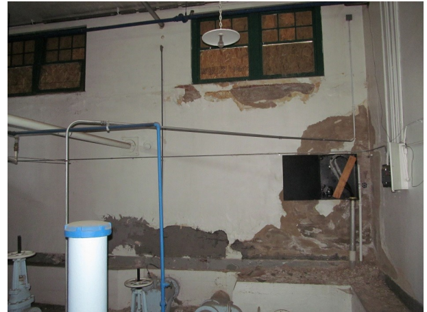
Deteriorated wall finish at basement
