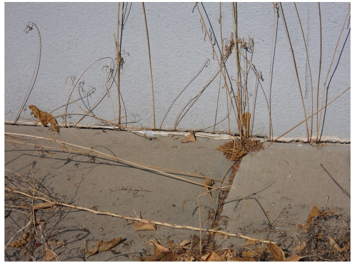
Deteriorated sealant joint at grade/base of wall
