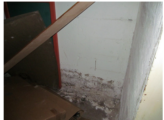
Water damage at basement storeroom
