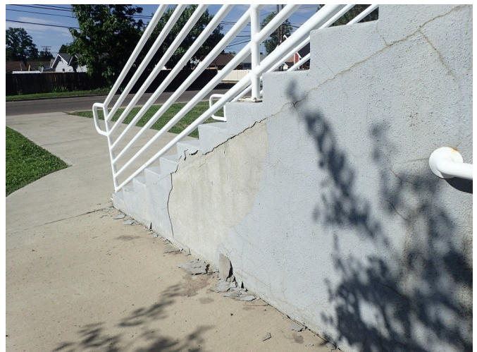
Parge coat at stairs
