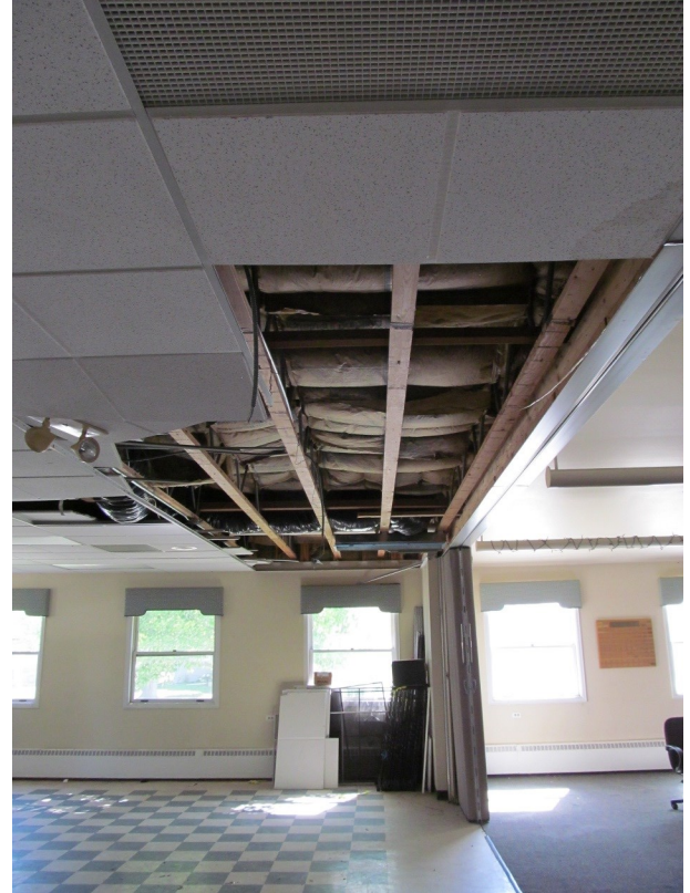
Ceiling damage at dining room
