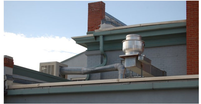
Kitchen hood exhaust and make-up system in 2024
