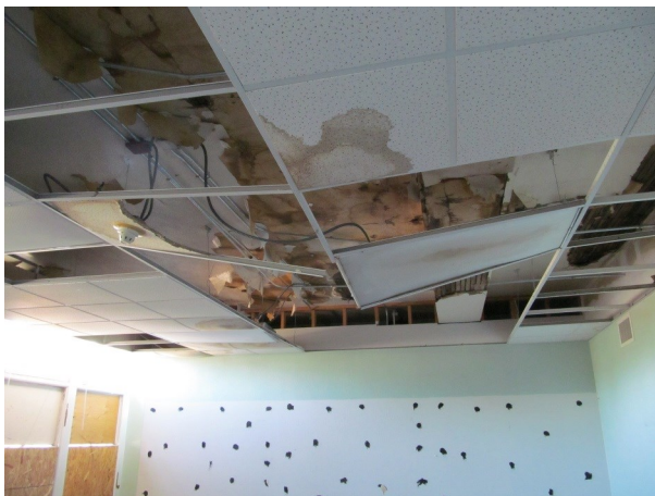
Ceiling damage at upper level
