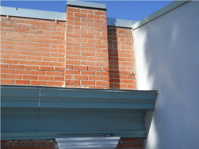
Deteriorated mortar at original building
