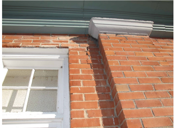
Deterioration of mortar joints
