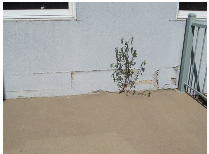
Cracks in EIFS at 1986 addition
