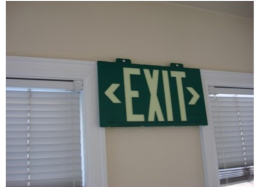
Non-illuminated exit sign
