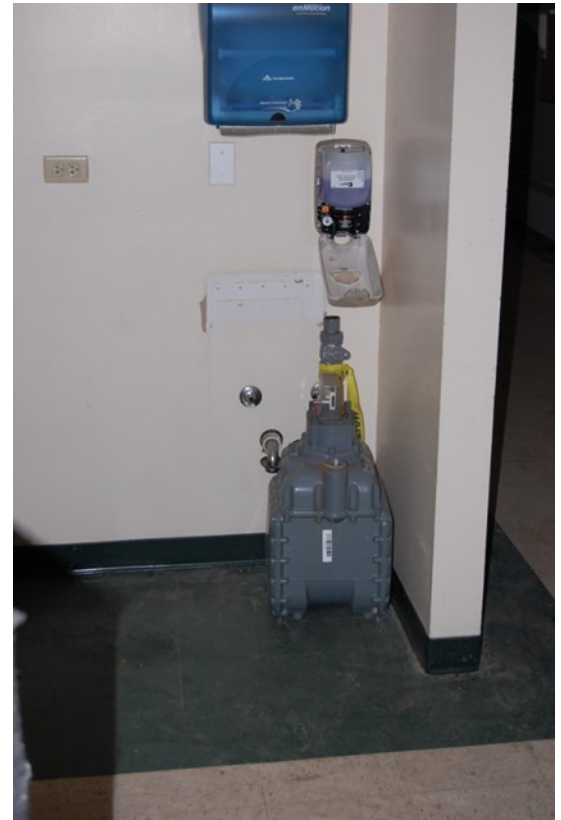
Plumbing fixture in 2024
