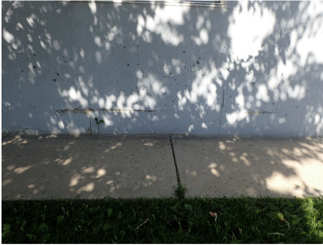
Cracks in exterior stucco
