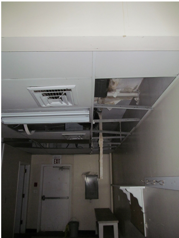
Water-damaged ceiling tiles at kitchen
