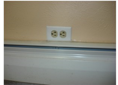
Receptacle above baseboard heater
