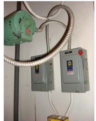
Mechanical equipment disconnects – kitchen mechanical room
