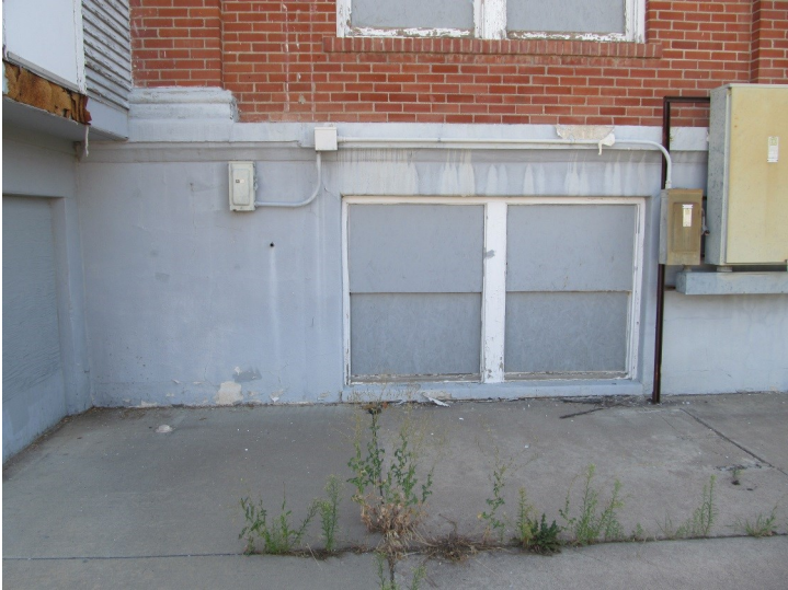
Damaged parge coat at west elevation
