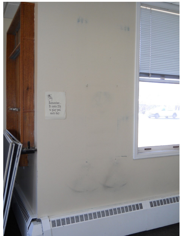
Damaged walls at billiards room
