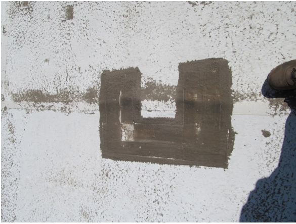
Defective patch at original building roof
