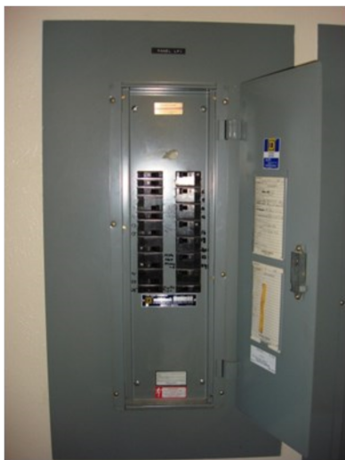
100A panelboard 'LP1'
