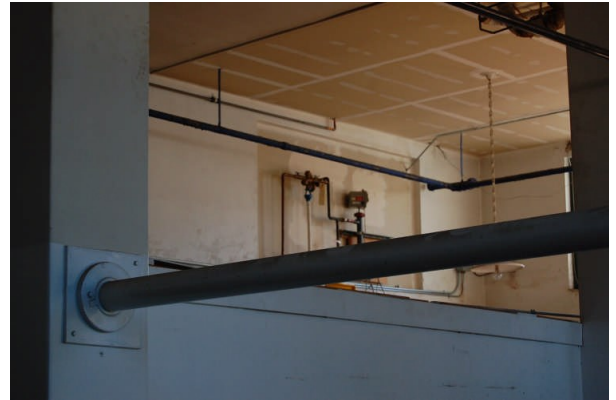
Domestic water backflow device in 2013
