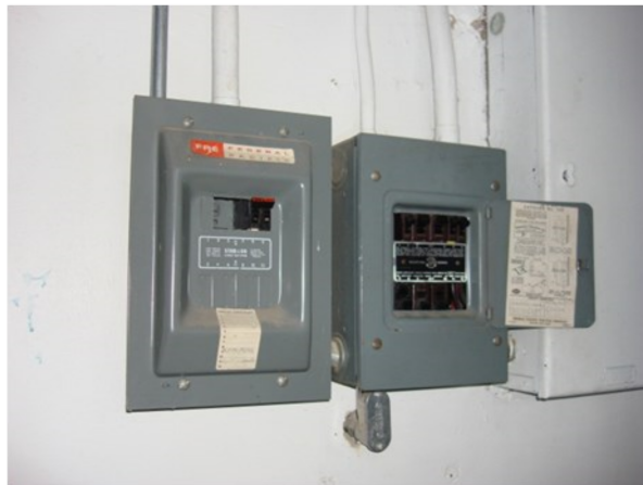
100A panelboard (basement)
