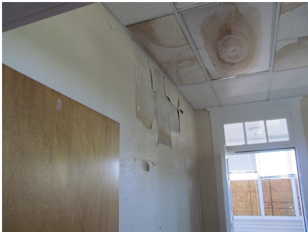
Drywall damage at upper level
