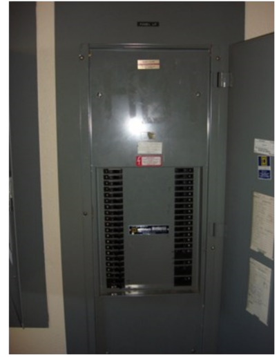
400A panelboard 'LP'
